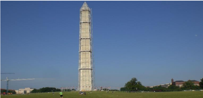
Washington Monument damaged after 2011 earthquake, closed and covered in scaffolding for repairs. (photo by Jade Phoenix Pence .)
